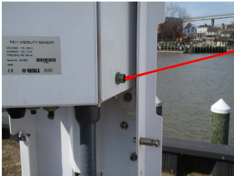
Figure 3. Visibility sensor maintenance port with dust cap removed.
